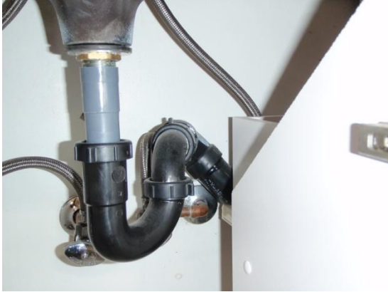
The drainage piping in the master bathroom sink cabinet is an improper design.
