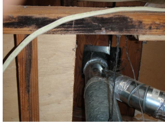
The distance between the flue and combustible materials is insufficient at the roof.
