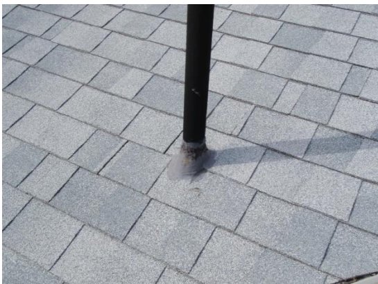
The flashing at several locations at the rear addition is not installed in accordance with best industry practices.
