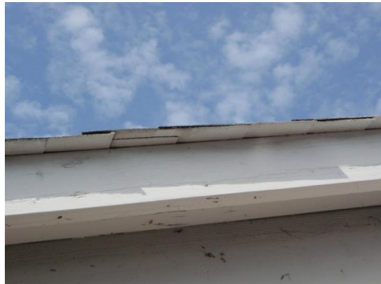
Edge flashing is not provided at the front, front north and rear south sides of the building.
