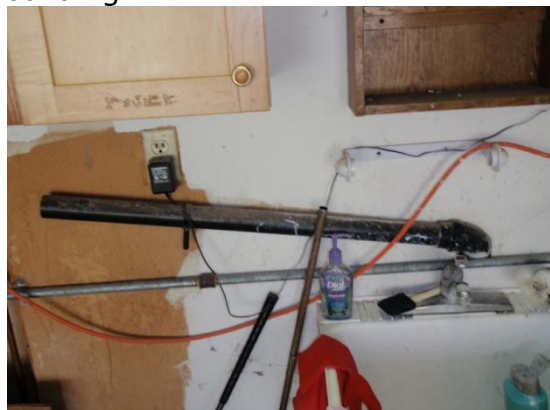
The washing machine drain is an improper design.
