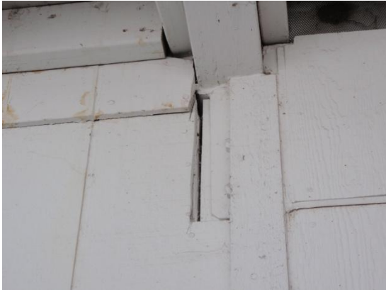
The siding is not sealed around the framing at the rear north side of the building.
