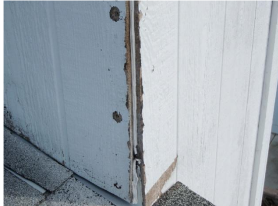
The chimney trim is loose and missing.
