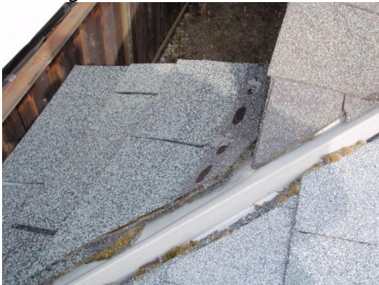
The roof covering is improperly installed at several locations.
